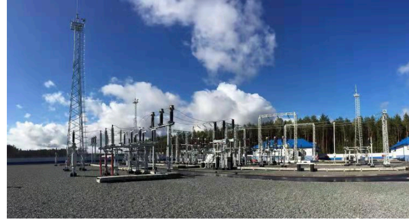
Belarus transmission line project
