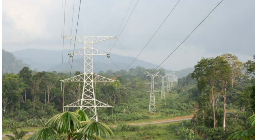
Transmission Line and Substations for Djibloho Hydropower Plant, Equatorial Guinea
